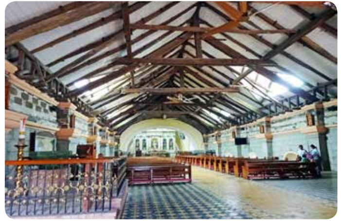
Bacolor Church is named for San Guillermo, the patron saint of Bacolor, Pampanga. Originally built in 1576, the church was destroyed by quake in 1880 and rebuilt 5 years later. In 1995 lahar flow from Mt Pinatubo engulfed the church, filling half of its 12-m height and forced the town's 50,000 residents to evacuate. The image shows the new floor of the church, with tiles laid over the lahar that half fills the original structure.
