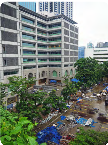
Looking down at the front of the new atrium, with the finishing in progress.
