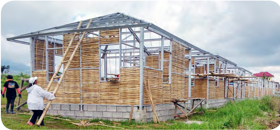
Houses built using a new earthquake- and typhoon-resistant design with steel posts anchored to a cement slab foundation.
