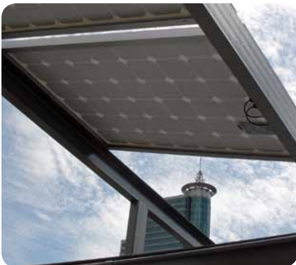
Solar panels on the roof of the new car parking building.
