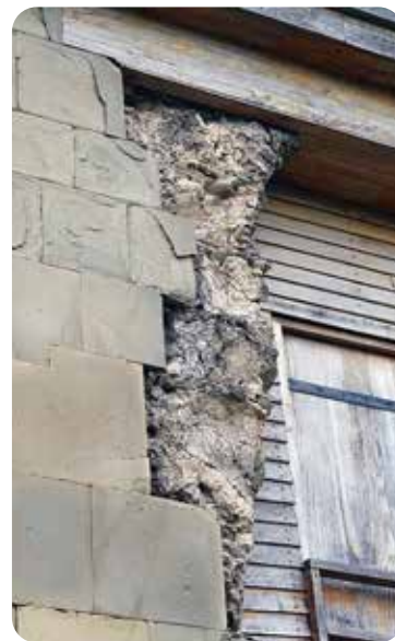
Evidence of Jvari's need for the ongoing restoration, and a glimpse of how the 1600-year-old structure was built.
